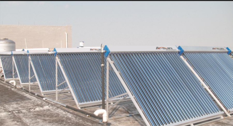
Solar Project in South Korea
